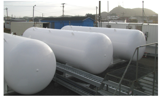
Hydrogen storage tanks
